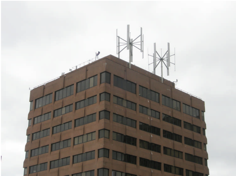
Figure 4. Marine Board Building, Hobart. Showing two of the original four 12KW Muce Vertical Axis Turbines
